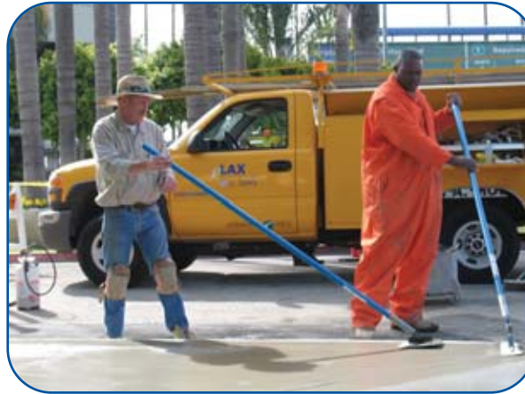
Construction and Maintenance Division cement finishers Tony Carrier and Robert Houston put final touches on project.
