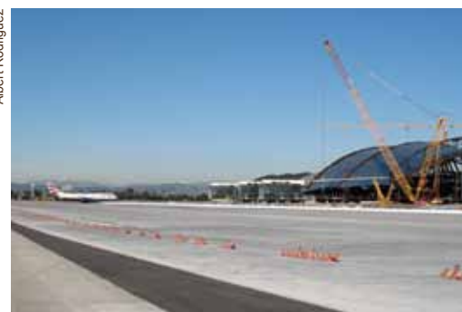
Taxilane S recently opened for aircraft operations, facilitating movement between the north and south runway complexes. The aprons or borders will be completed by early summer.
