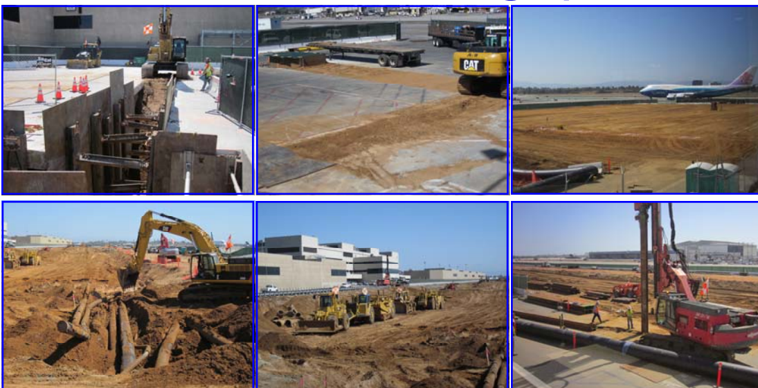
Construction Photographs Clockwise From Upper Left: ➤ Utility Trench at Gate 106 ➤ Utility Trench at Gate 119 ➤ Interim West Busing Terminal Engineered Fill ➤ Shoring for Excavation ➤ Concourse & Core Excavation ➤ Abandoned Fuel Pipe Removal
