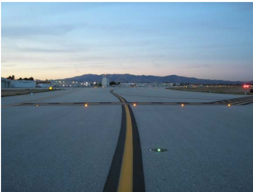
In-pavement Runway Guard Lights
