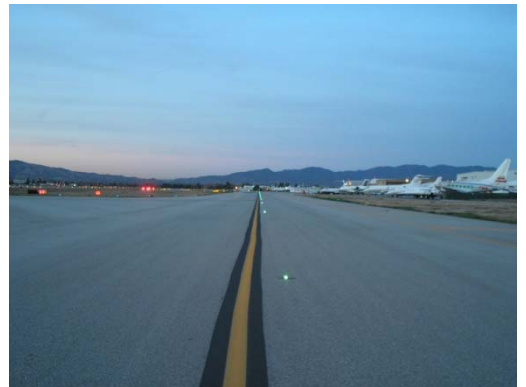
Taxiway Centerline Lights
