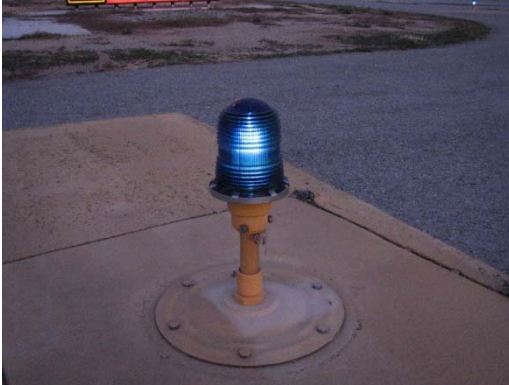
Taxiway Edge Light (elevated)
