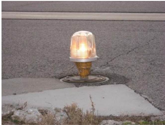
Elevated Runway Edge Light Fixture
